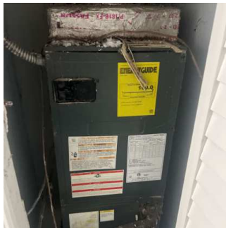
Air Handler (1/2) 09/05/2025 12:33 PM
