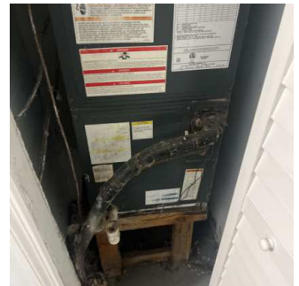
Air Handler (2/2) 09/05/2025 12:33 PM
