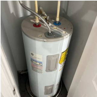
water heater 09/05/2025 12:46 PM
